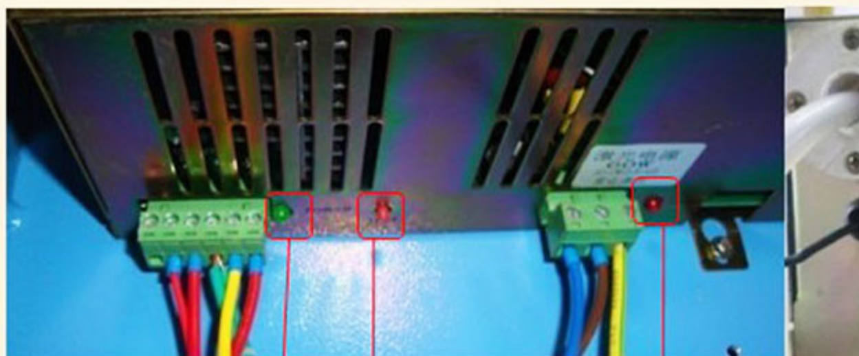
Power indicator lamp
